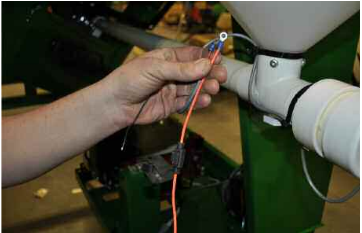
Crimp eyelets onto the red wire and fuse, then tighten onto the switch (below).
